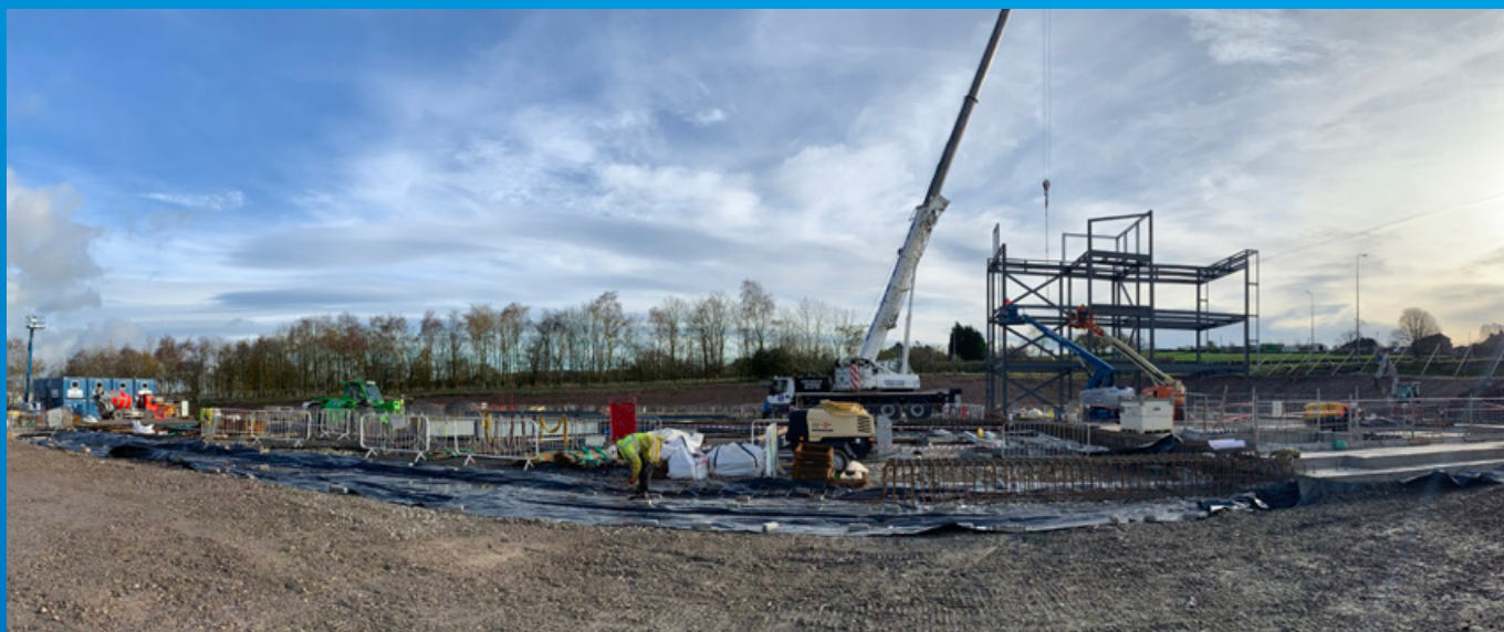
Construction is underway on the £20m University of Sheffield AMRC North West in Lancashire as the steel frame of the building begins to take shape.
